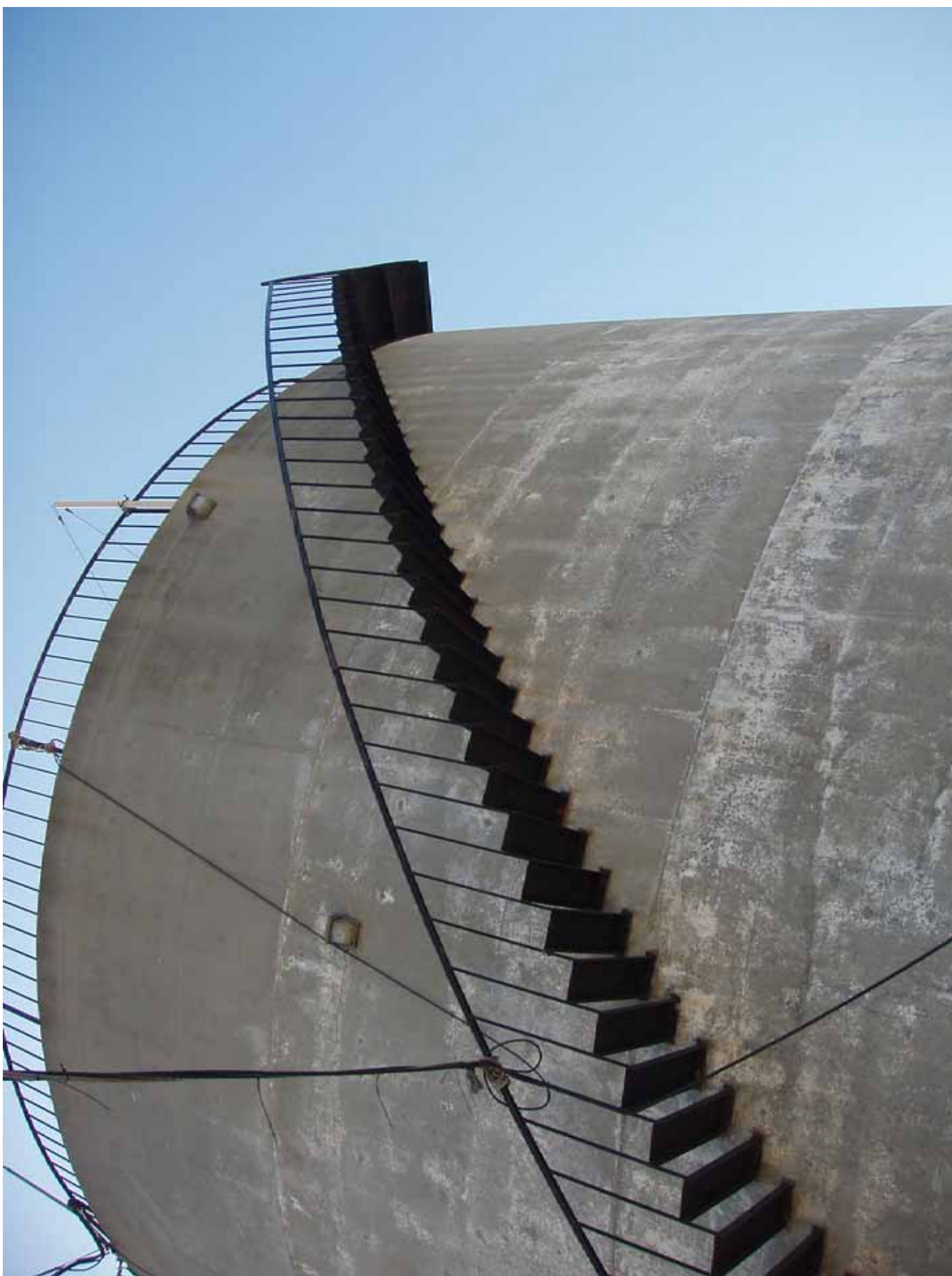
B-12 Water Storage Tank On Top Of Terminal Hill
