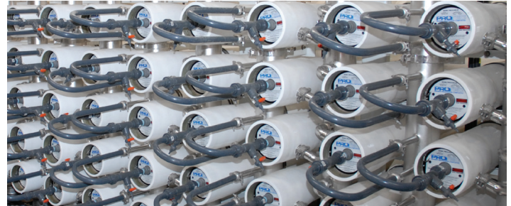
Recycled Water is highly treated by microfiltration and reverse osmosis at the City's Terminal Island Water Reclamation Plant. This water is injected into the Dominguez Gap Seawater Barrier to protect groundwater supplies from seawater intrusion.
