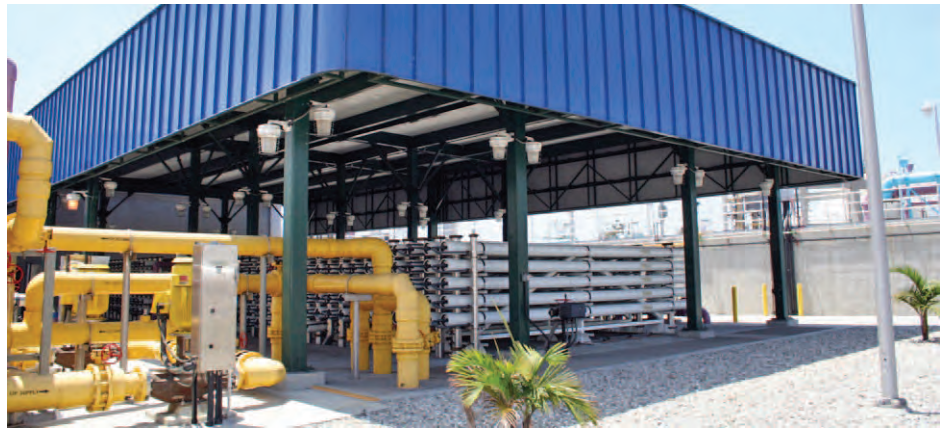
AWPF at TIWRP producing highly purified water
