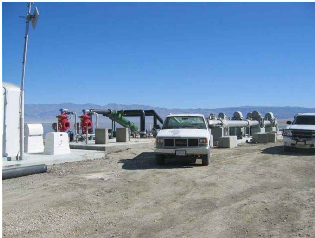
Figure 3 Existing Turnout on Owens Dry Lake
