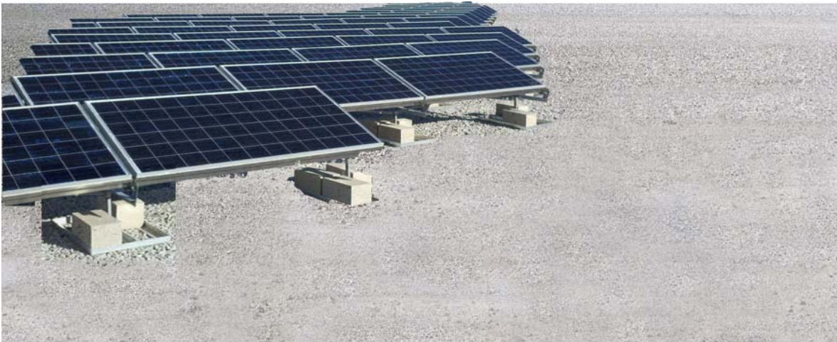
Figure 7 Solar Panels on Dolomite Gravel Cover
