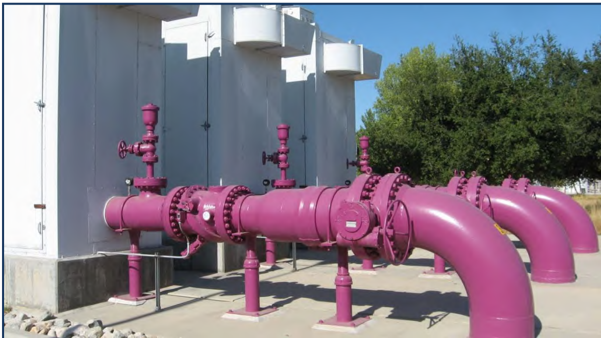
Figure 6: Balboa Pump Station
