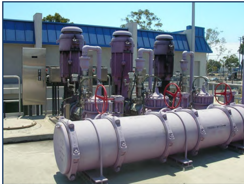
Figure 3: Product Water Pump Station
