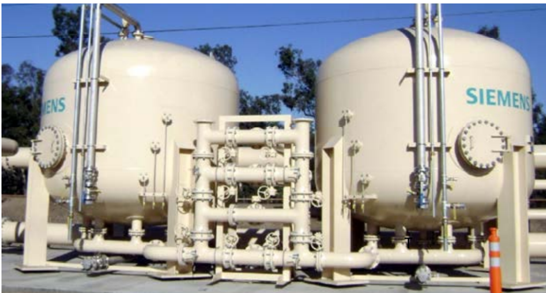
Typical Liquid Phase Granular Activated Carbon Vessels
