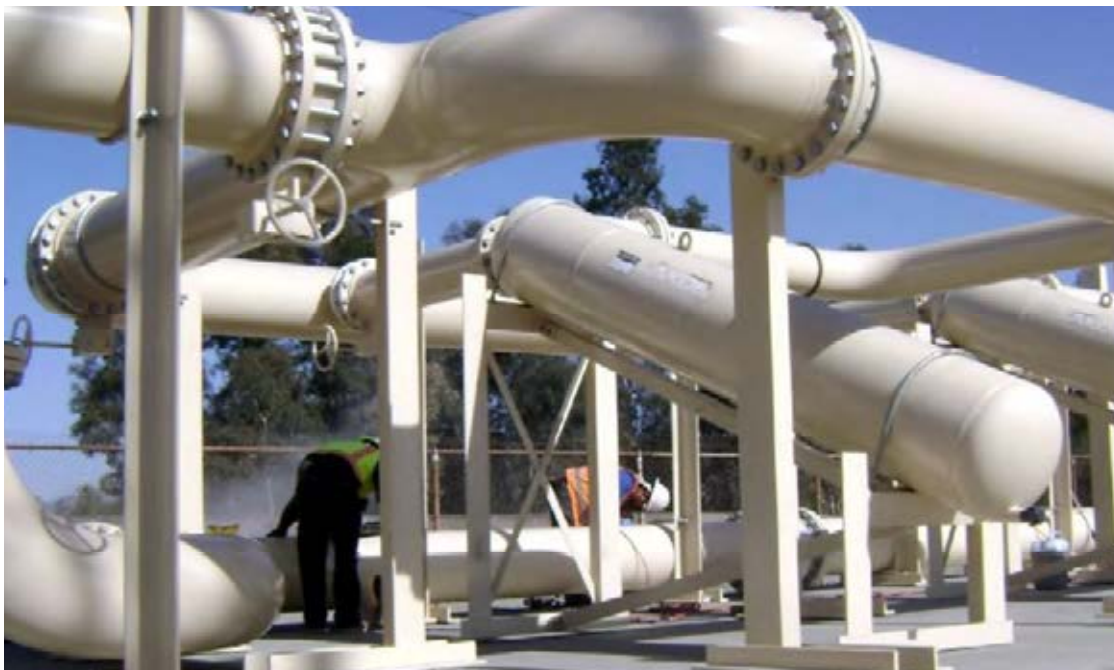
Typical Pre-Filtration Unit
