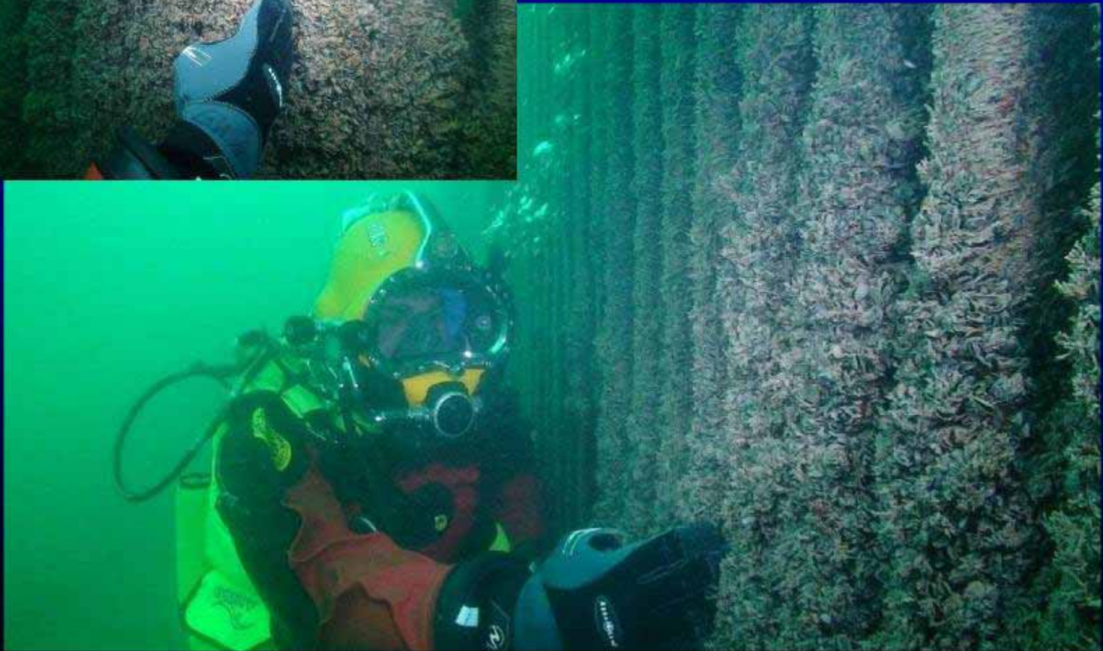
Mussels on Water Intake Screen – Lake Havasu
