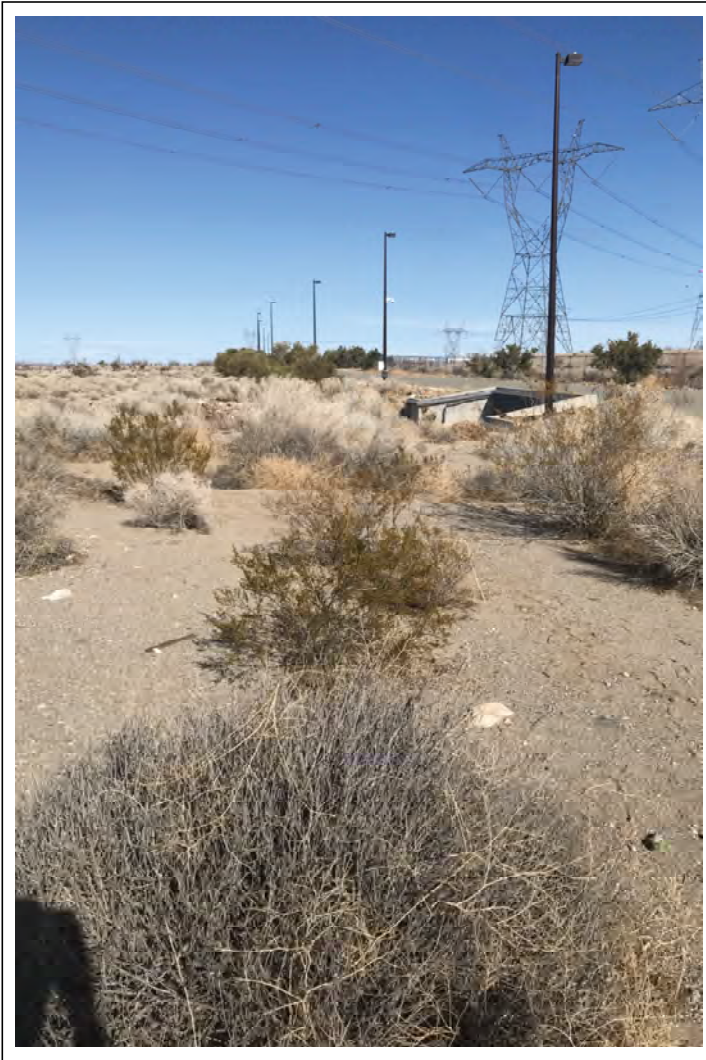
Photo K - View of the culvert that conveys Drainage 6 beneath Aster Road.
