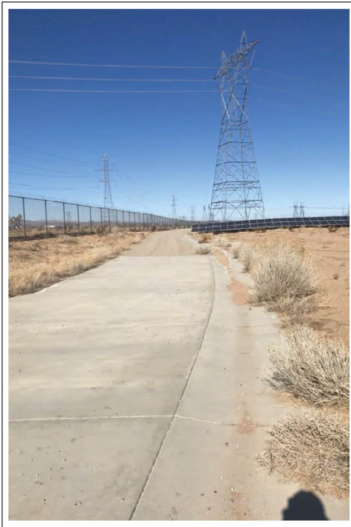
Photo E - View to the north along Drainage 11 which flows out of a culvert and along a ribbon gutter before joining Drainage 2 to the north.
