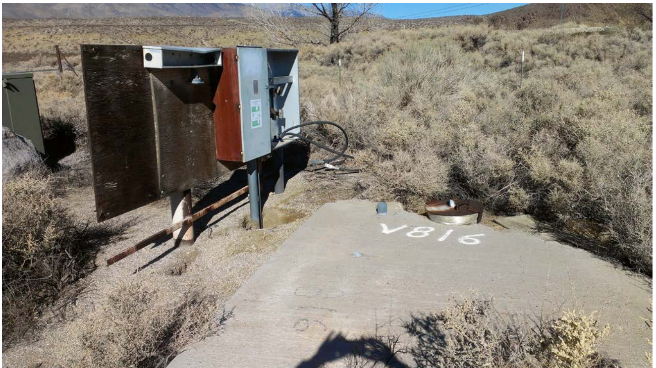
Well V816 and the adjacent, unused electrical junction box/panels (one is far left). Power to the well pump will be controlled from the upgraded panel components that will be installed at this location.
