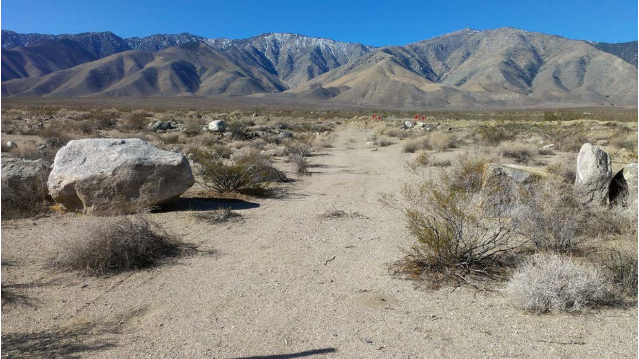
This is the existing dirt access road that will be excavated to allow placement of the pipeline connecting V817 to the First Los Angeles Aqueduct. Pipeline will deliver the pumped water to a concrete access box (in this picture, marked by barricades along the right side of the road in the distance)
