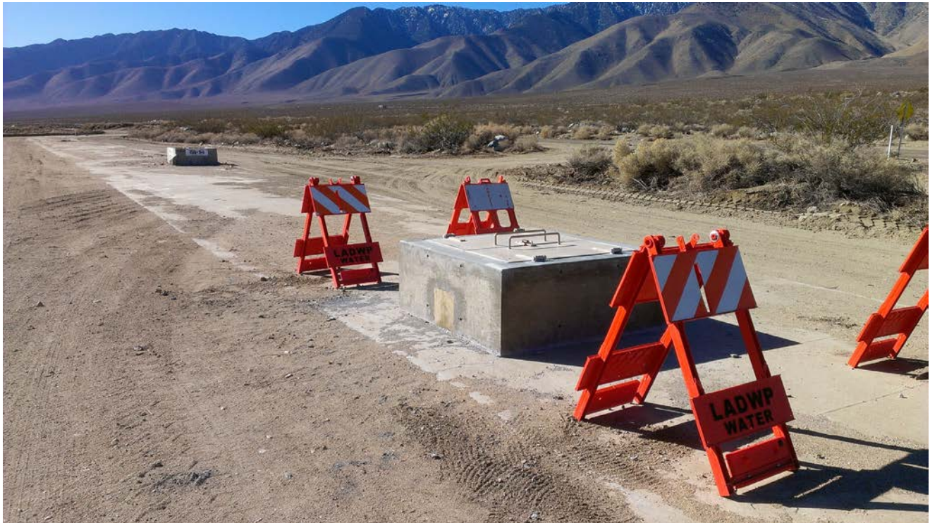
Concrete access box atop the concrete cover for LAA1. Pipeline from well V817 will connect to this access box to deliver pumped well water.
