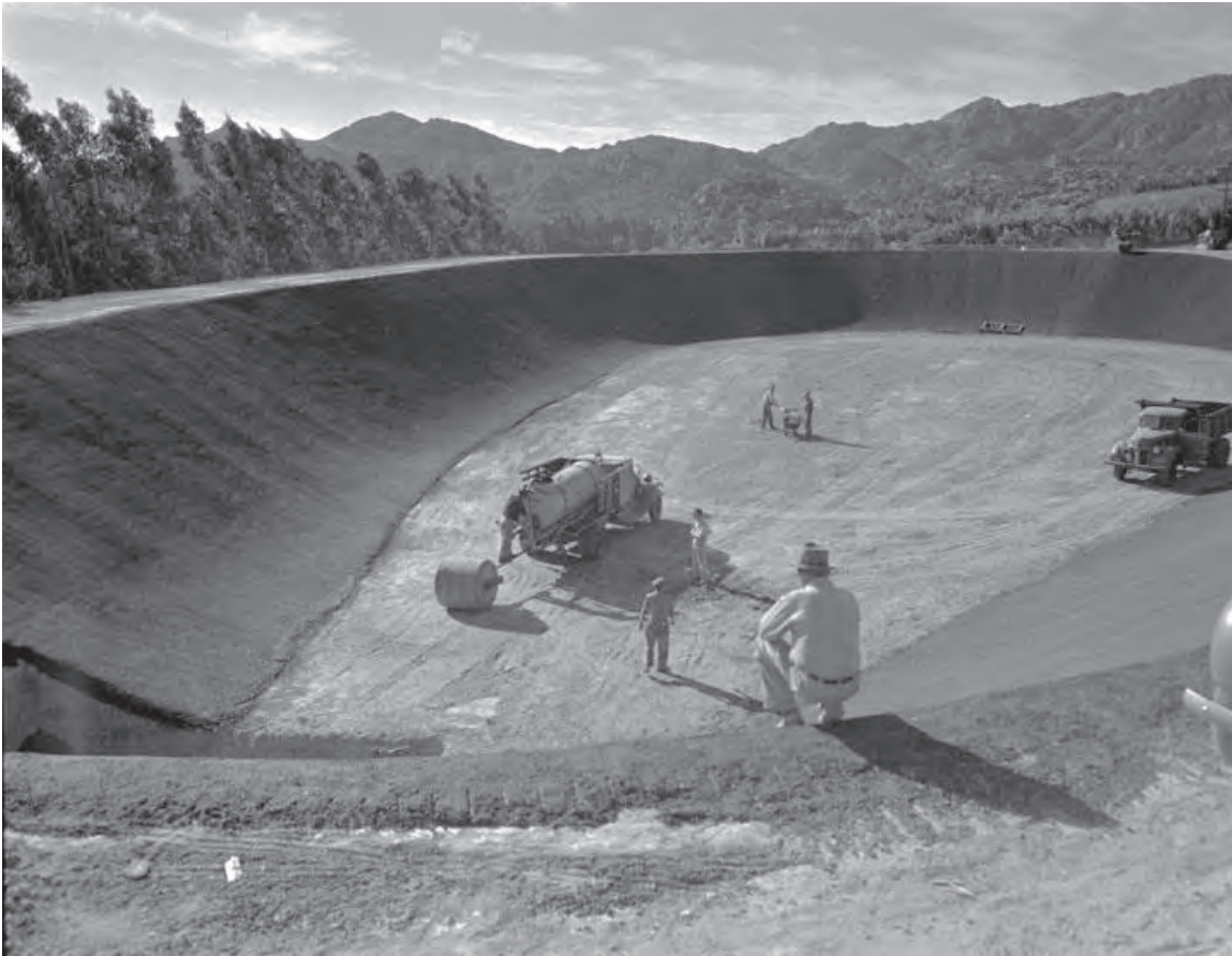
Figure 8. Photo demonstrating the roller compaction technique pioneered at the De Soto Reservoir, 1942, looking east. (LAPL 1004960, also held by LADWP Record Center)
