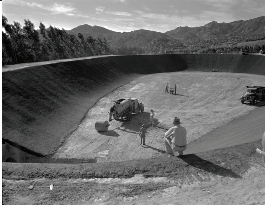
Figure 5. Photo demonstrating the roller compaction pioneered at the De Soto Reservoir, 1942, looking east. (LAPL 1004960, also held by DWP Record Center)
