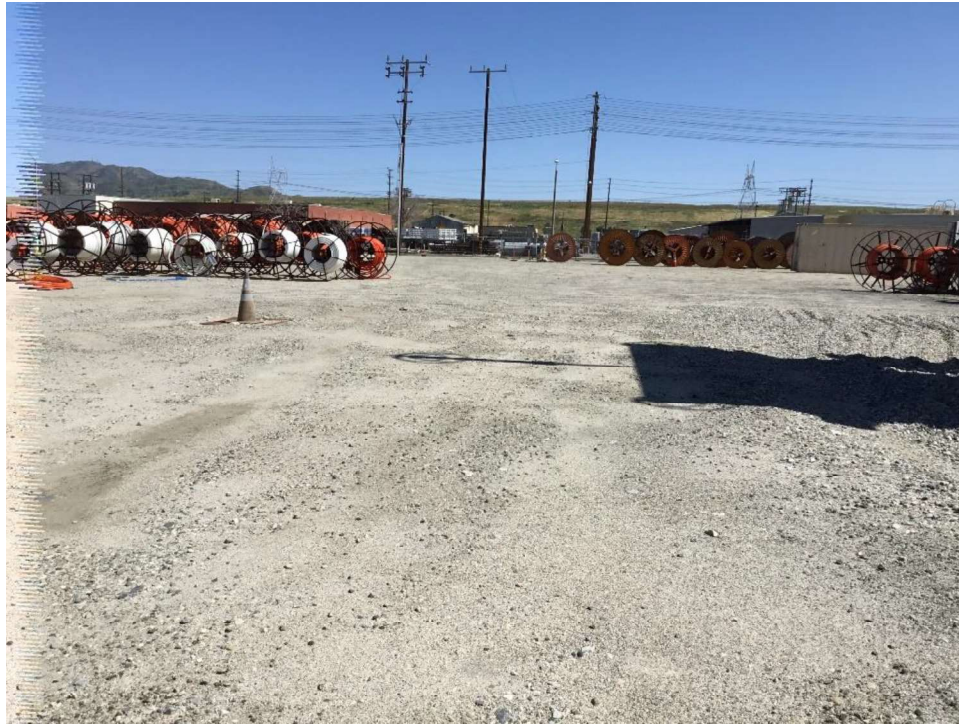
Figure 14. Overview of area surrounding the demolished cooling towers, view facing south (IMG_3284)
