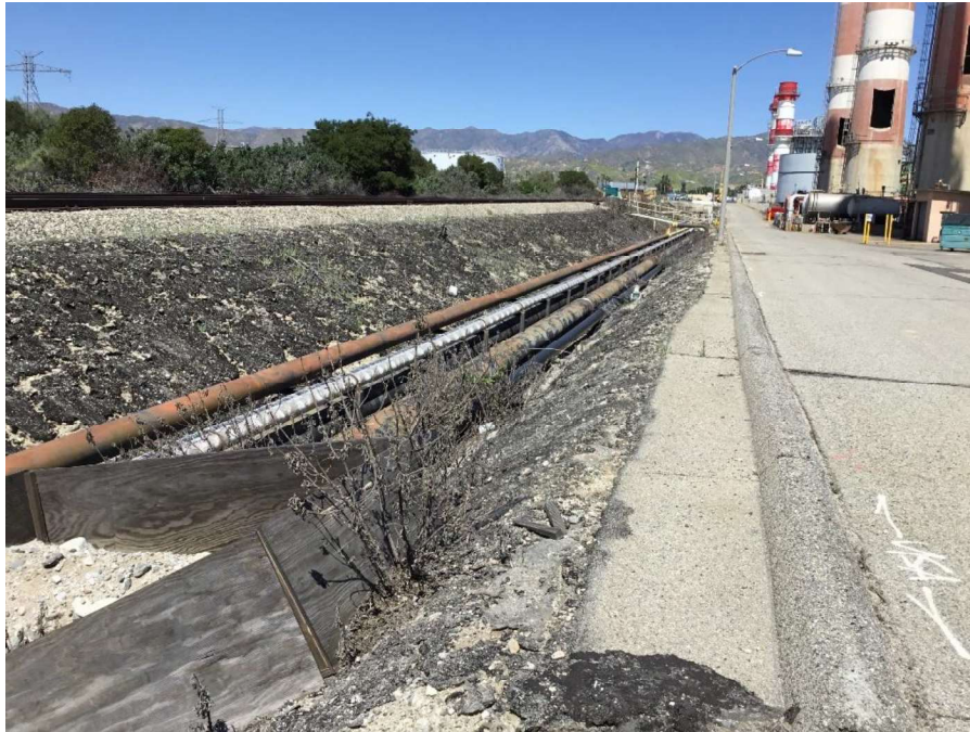
Figure 12. Overview of pipeline to the north of the Units, view facing east (IMG_3226)
