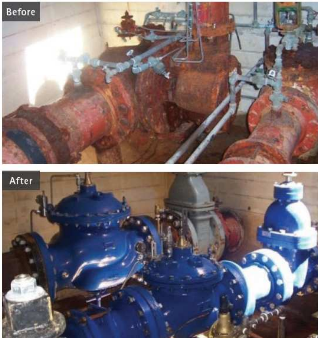
Figure 24: Pressure Regulator Before and After Replacement
