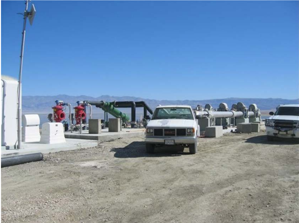
Figure 3-7 Existing Turnout (T1A-2 DCA) on Owens Lake
