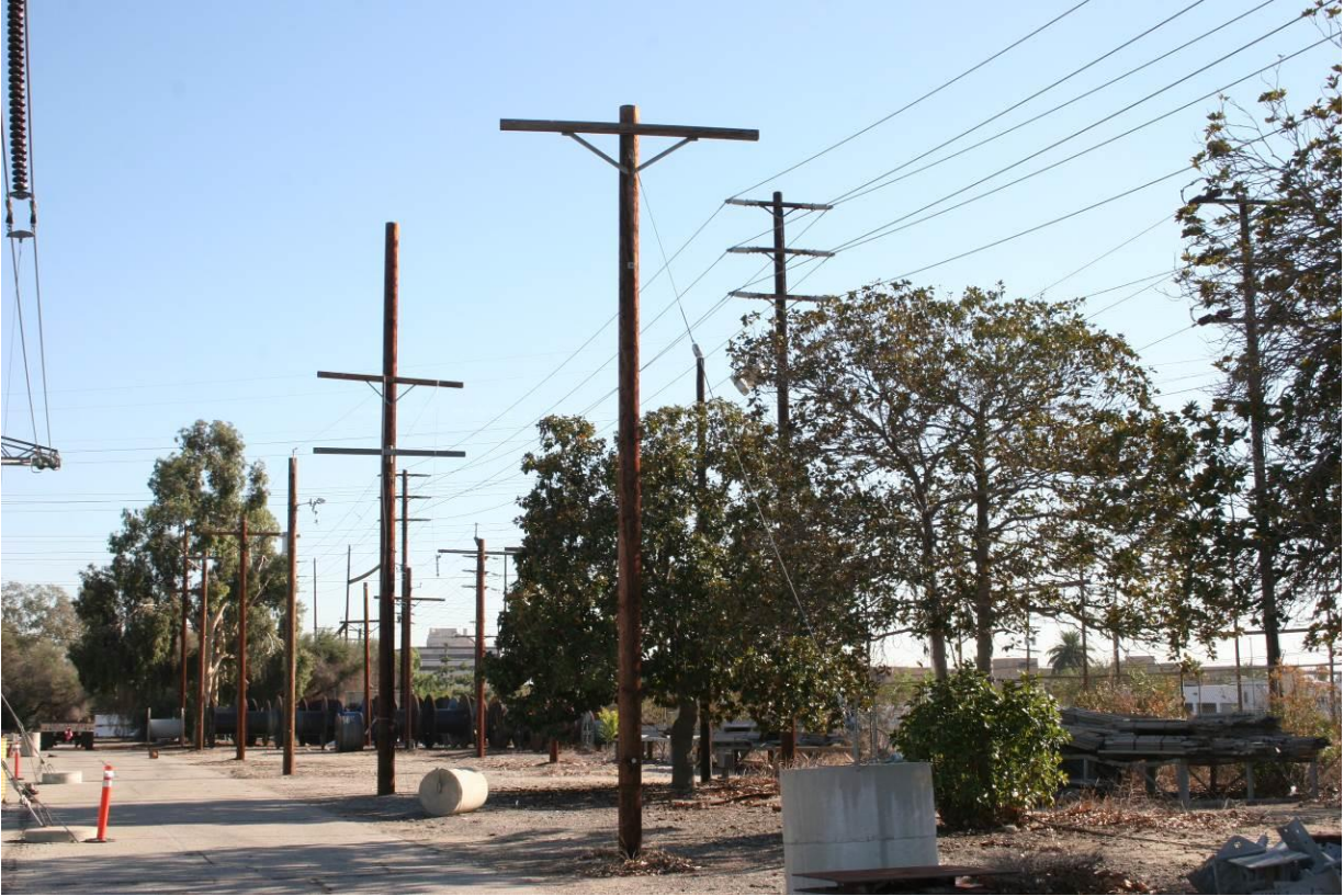
Plate 9. Inoperative Wooden Power Poles, View Southeast.
