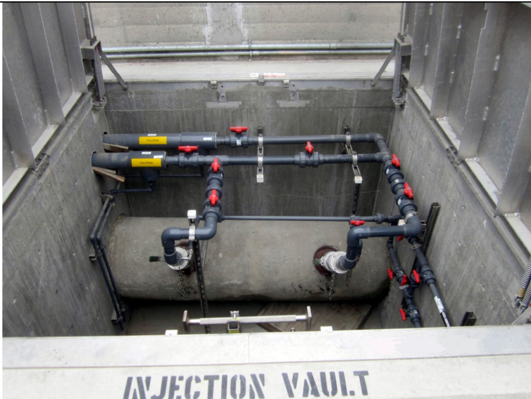
Photo B Typical Hydrogen Peroxide Injection Vault
