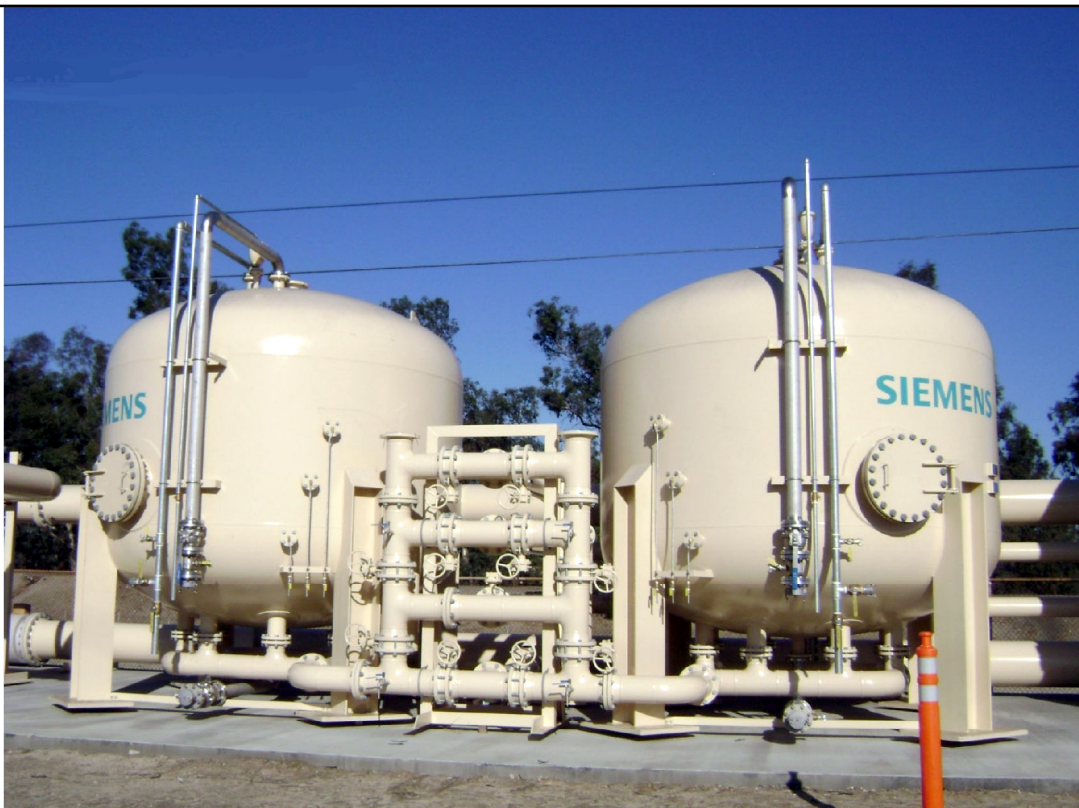
Photo B Typical Liquid Phase Granular Activated Carbon Vessels
