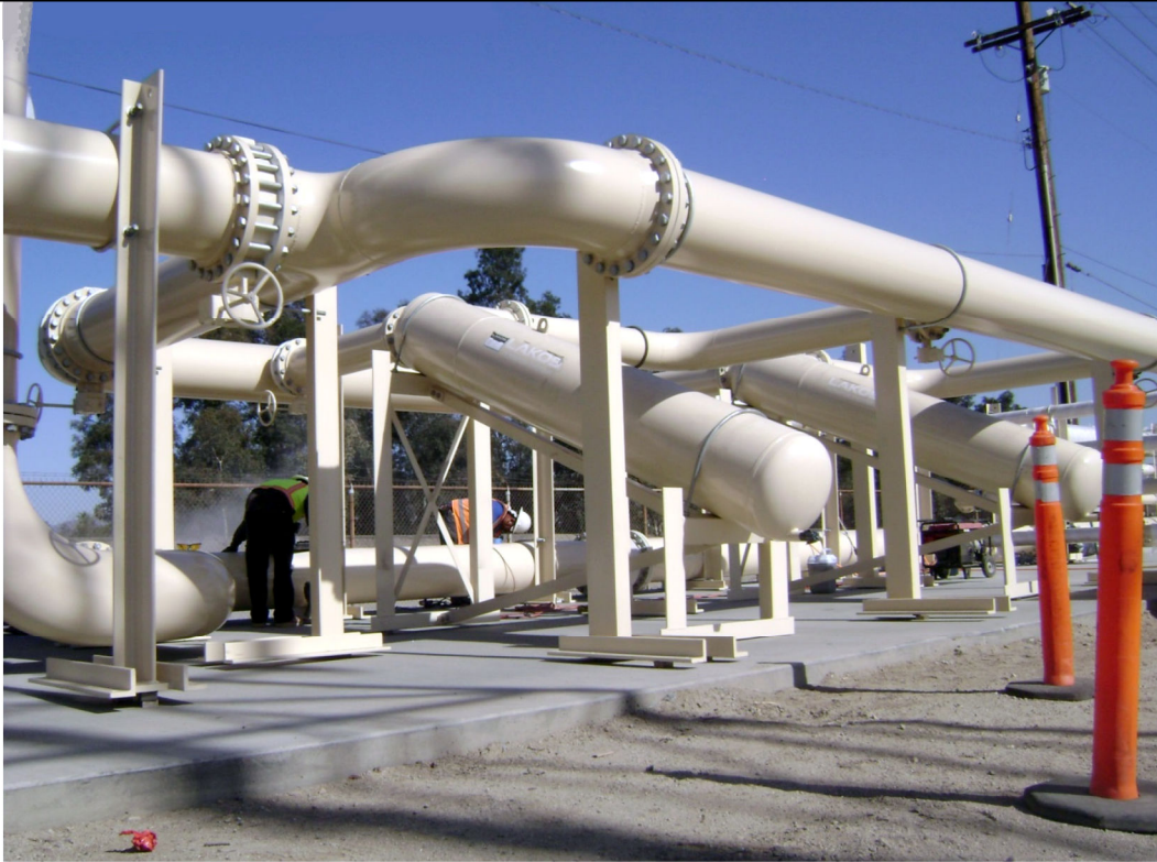
Photo A Typical Prefiltration Unit (Sand Filter)
