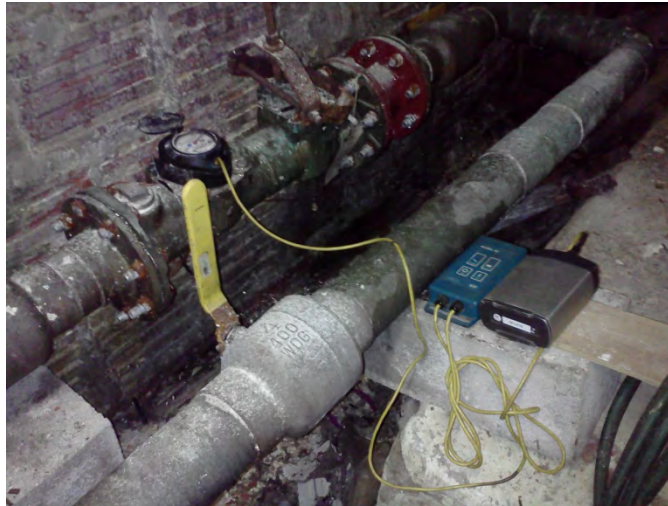
Figure 88: Meter-Master Installation and Data Logger – TRO Ave of the Arts
