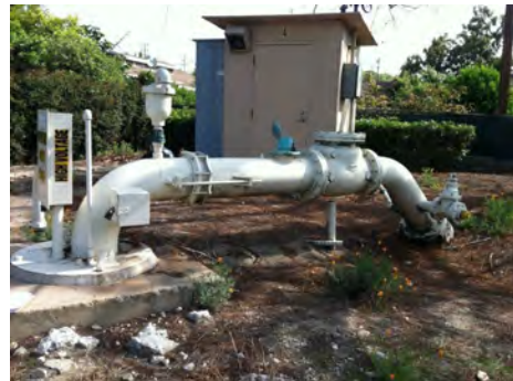
Figure 65: Pollock Well Site Visit
